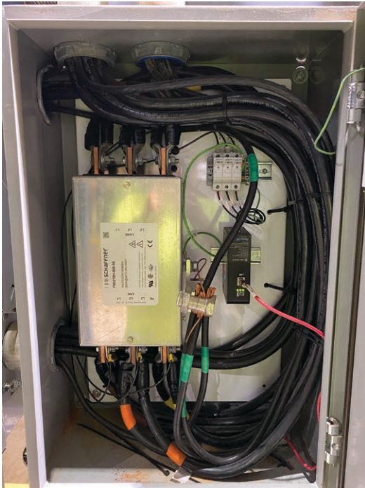
Figure: 6-6 - Improper Installation of System
